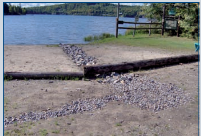
The drainage improvements implemented at the site work to divert polluted water from the roadway to soak into the ground instead of eroding sediment from the beach and polluting Back Lake.
