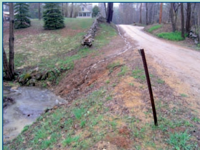
With the spring rains often comes polluted roadway runoff. A vegetative buffer or an infiltration trench along this roadway would help minimize the amount of sediment and other pollutants flowing into the stream.
