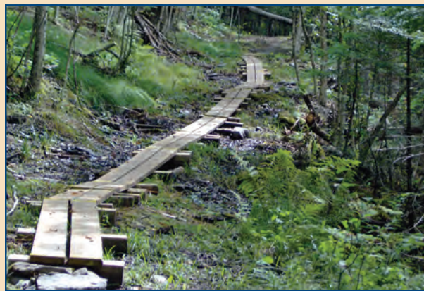
The LCC crew in Pittsburg constructed an extensive boardwalk along a popular but muddy hiking trail.
